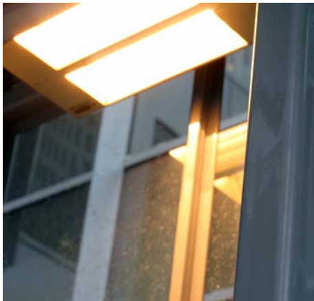
Figure 29: Heated lamp for transit users
